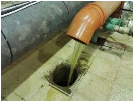
Disc filters discharge
